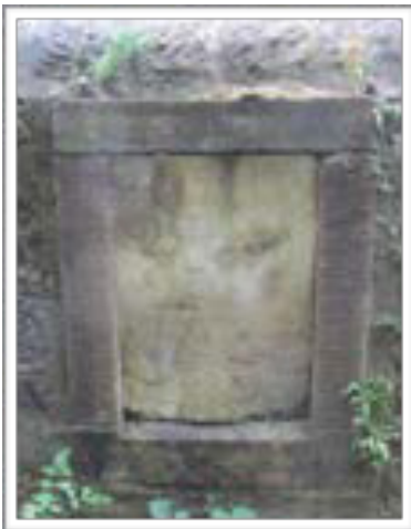
Inscription panel missing
