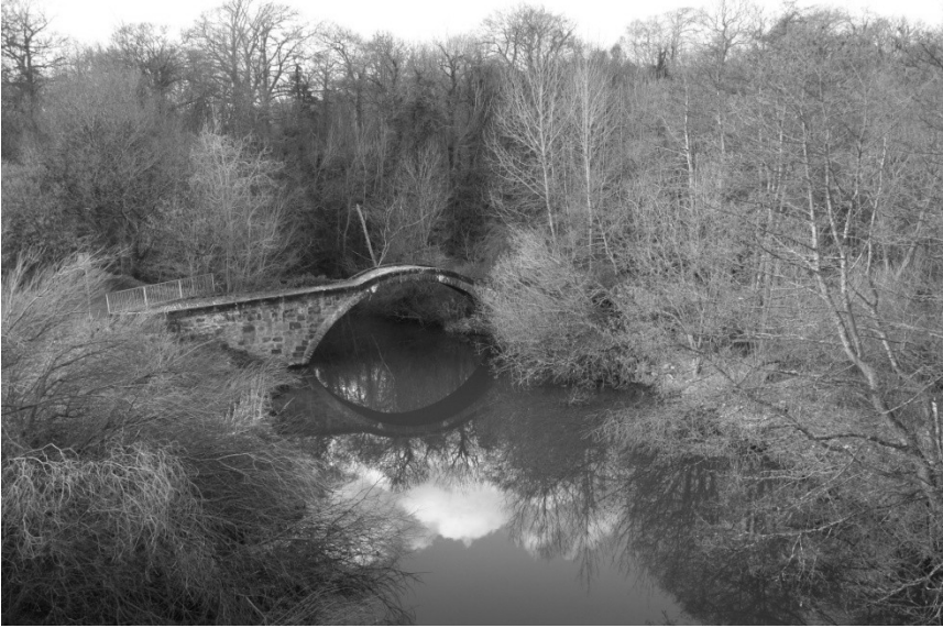
Seventeenth Century packhorse bridge known locally as the Roman Bridge adjacent to the site of the Roman Fort at Bothwellhaugh
